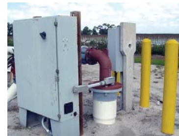
Figure 3. A 25-hp pump draws water from a 60-ft deep well at the Harris Moran Research Station. The well's plastic casing does not provide a natural grounding path. That fact, plus poor grounding elsewhere on the station led to several pump failures.
