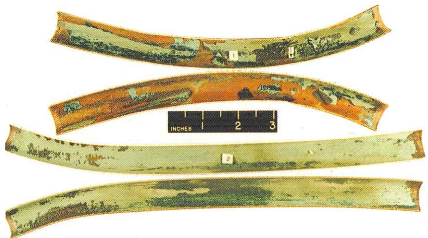
PHOTO B. Hydrogen-sulfide-induced pits overlaid with friable green to black tubercles of copper-corrosion products. Loosely adherent and porous layers of copper sulfide have broken free from the upper two tube half-sections.
