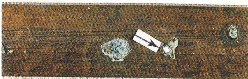
PHOTO H. Chemistry-related-hot-water-induced pits covered with friable tubercles of green copper-corrosion products. Loosely adherent layers of brown hydrated hematite deposits cover black cupric oxide on the water-side surface of a hot-water line.
