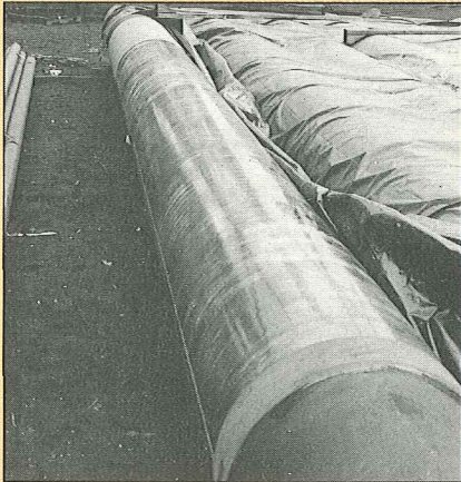
One of the Eureka jacket's 60 conductors is coated in the splash zone with Mark Tool's Bio-shield, a thin Cu-Ni alloy bonded to the pipe with an elastomer.
