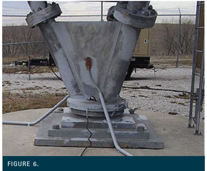
FIGURE 6. One of two original AWG #2 copper ground leads at the tower base (foreground, bare wire) were augmented by three new 250-kcmil tinned copper conductors (two shown, in protective sleeves).
